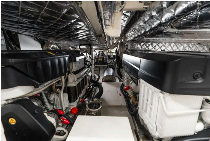
Engine room of 2024 Cranchi Sessantasette 67 yacht, showcasing advanced machinery and insulation.
