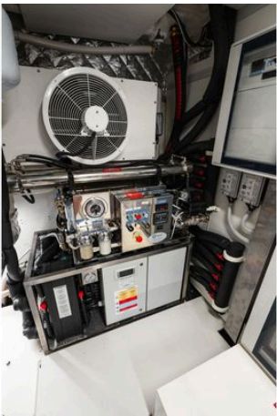
Engine room of 2024 Cranchi Sessantasette 67 yacht, featuring advanced machinery and ventilation system.
